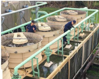
CDR Gumapas and CDR Yang shutting off valves to prevent 90,000 gallons of water loss per day in Bayamon, PR
