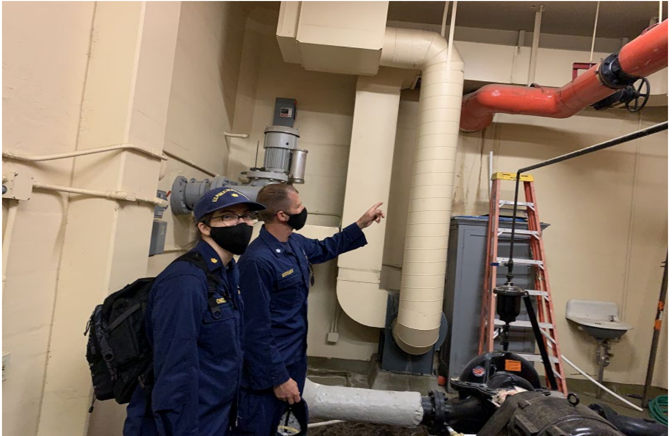
CDR Kesteloot and LCDR Dondzila evaluating the Hot Springs National Park main thermal water collection line at the overflow weir before the water enters into the first main water reservoir at ~147 degrees Fahrenheit.
