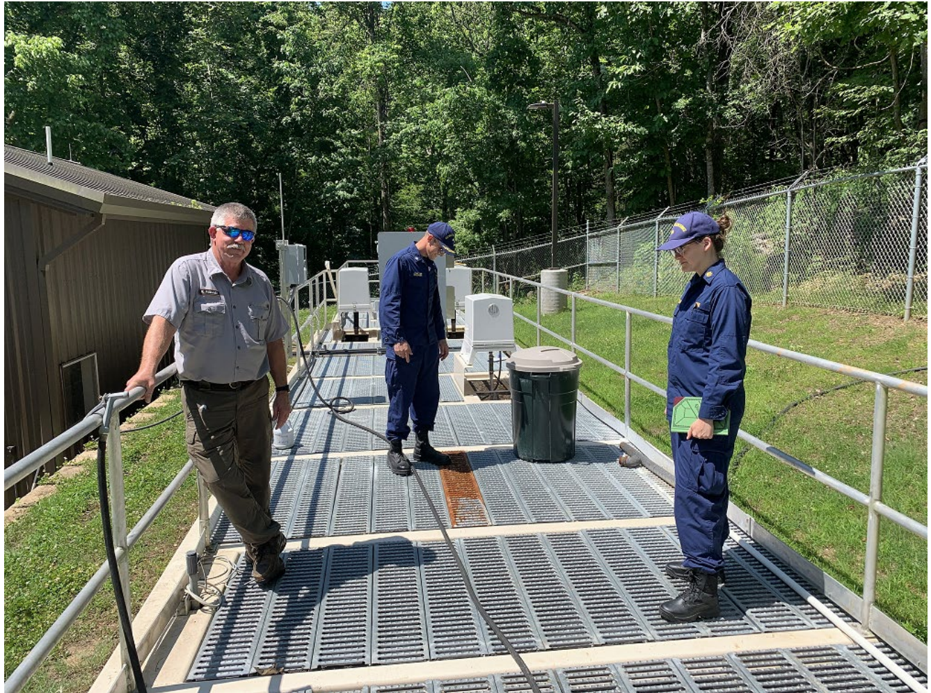
Robert Pugsley, CDR Kesteloot , and LCDR Dondzila on top of the new active sludge wastewater treatment plant at Buffalo Point in Buffalo National Riverway park . This plant was recently installed based on recommendations provided by National Park Service Office of Public Health.
