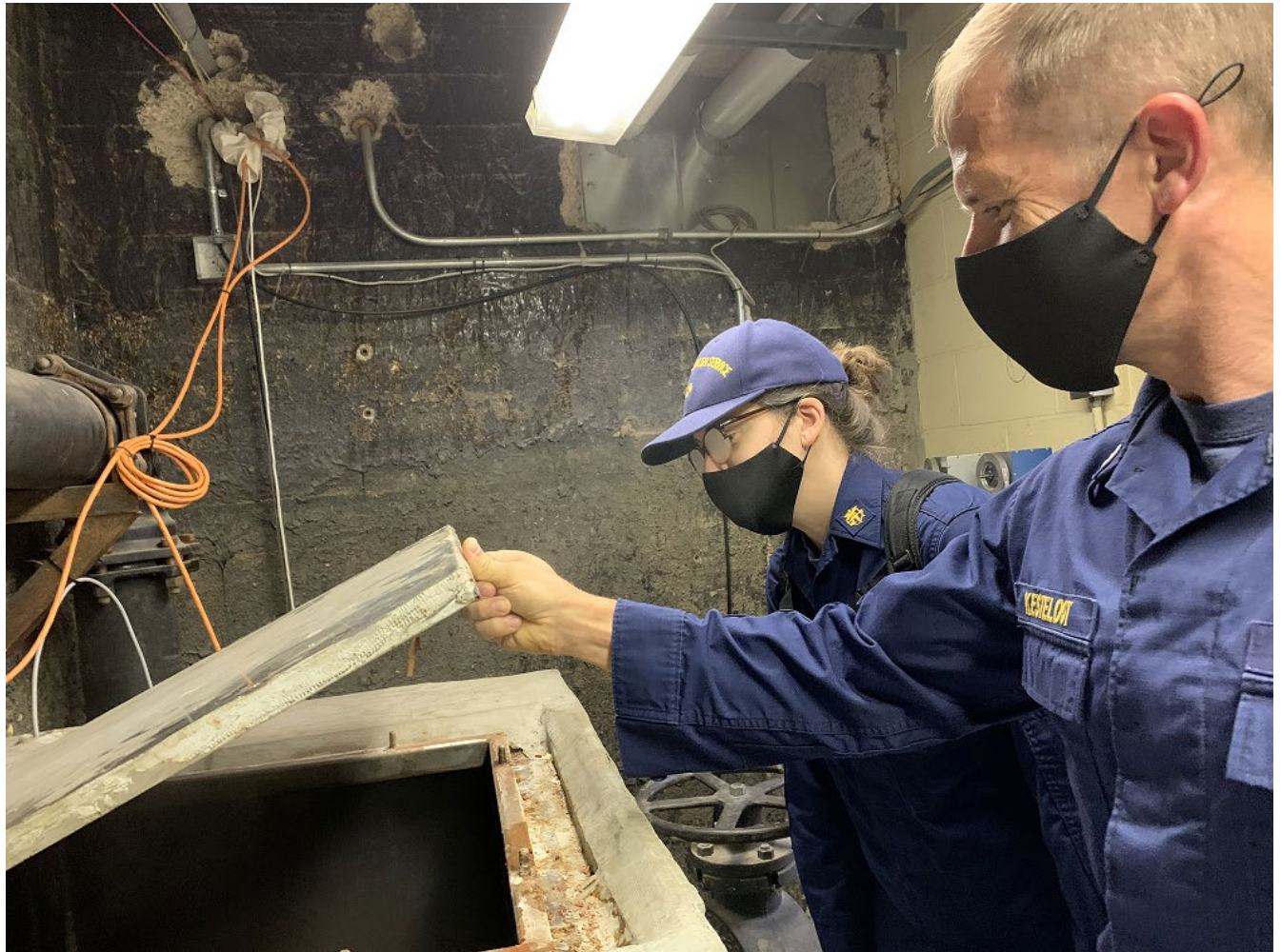
CDR Kesteloot and LCDR Dondzila evaluating the Hot Springs National Park thermal water systems' first set of booster pumps and controls. Note that the water is still about 145 degrees Fahrenheit at this point in the system.
