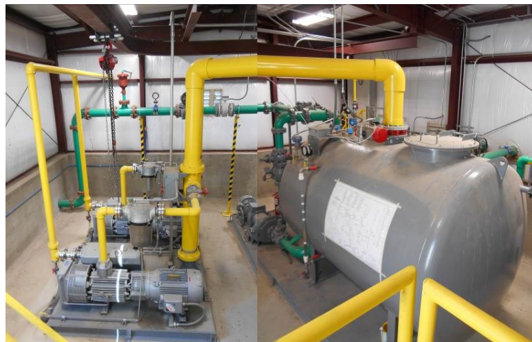
Inside a Vacuum Station
