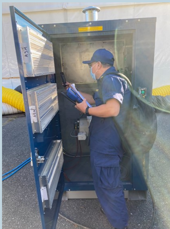
LCDR Qi evaluating an air handling unit that was servicing a shelter housing vulnerable population
