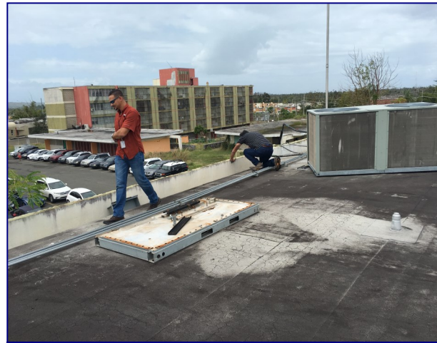
April 11, 2018 – Centro Pediatrico Mayaguez – displaced A/C units on rooftop; this was a common issue
