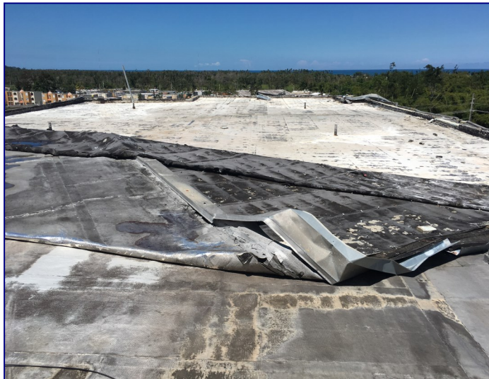
April 5, 2018 – Laboratorio Mayaguez – peeled back water proofing material on rooftop creating issues throughout the floors below
