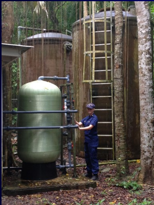
LTJG Kelly Hoeksema checks valve orientations on media filter tank at Trunk Bay's reverse osmosis plant, Virgin Islands National Park.
