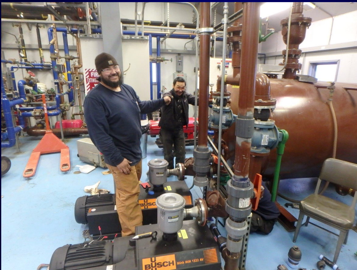
ARUC utility support engineer Michael Nabers (foreground) installing two oil less vacuum pumps in the community of Savoonga’s sewer plant, with plant operator Cedric Toolie in 2014.
